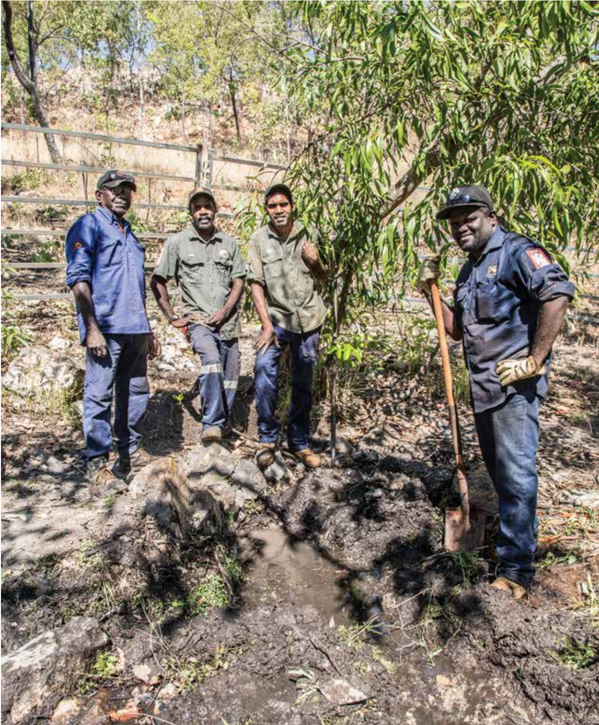
Above: Feral animals and weeds had blocked the sacred Gulin Gulin Spring at Bulman where old people used to gather to plan ceremony. In 2016 djungkayi Kenneth Murray and rangers installed a cattle panel fence to keep out feral animals. They cleaned the spring and removed gmelina trees. Following the next wet season the spring started running more strongly.
